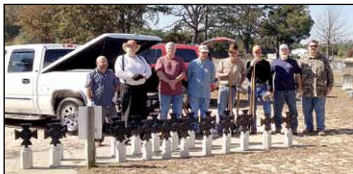
Members of the Colonel Stephen Jackson Chapter 295 MOS&B and members of the First In Secession Camp 1963, Chesterfield, SC, installed 22 Southern Iron Crosses at the Elizabeth Baptist Church, Mt. Corgan, SC.
